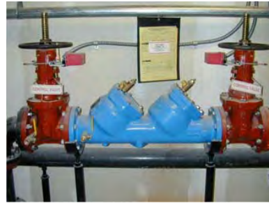
FIRE SPRINKLER SYSTEM
